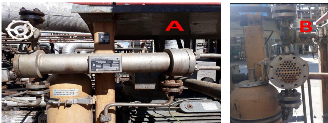
Fig. 2. A: Real shell and tube cooler of the circulation seal oil of the RFCC MCB pump that has been modeled B: Tube sheet of the heat exchanger.
